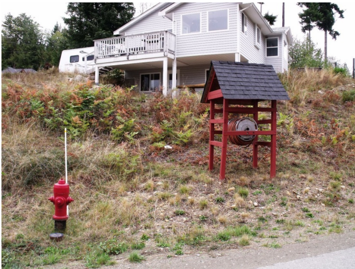
Photo 2 Dashwood Volunteer Fire Department hydrant and strata hose reel, Country Road in Little Qualicum River Estates.
