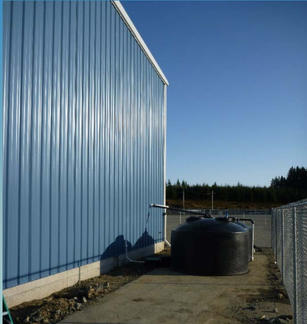
Two 1200 gal (5.5m 3 ) tanks
