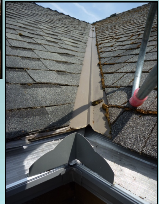
Diverters at Valleys
