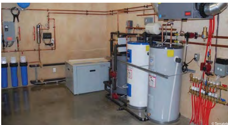
The grey box in the corner is the heat pump, the heart of a geexchange system. Red hoses for in-floor heating. Domestic hot water back-up tank (r), buffer tank and desuperheater for domestic hot water pre-heating (l).
