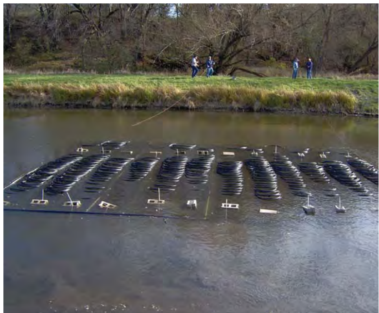
Pond loop being sunk. Length of pipe is sized to accommodate the home's heating and cooling requirements.
