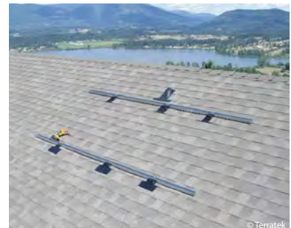
Flush-mount roof racking system for solar collectors.
