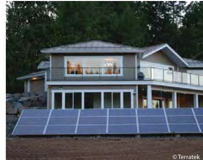
Six kilowatt ground-mount installation, Nanaimo, BC.
