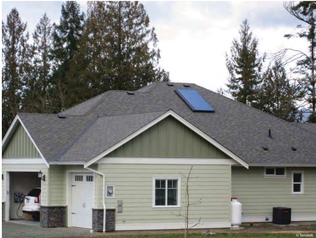
Single collector solar hot water system on new home in Duncan, BC.
