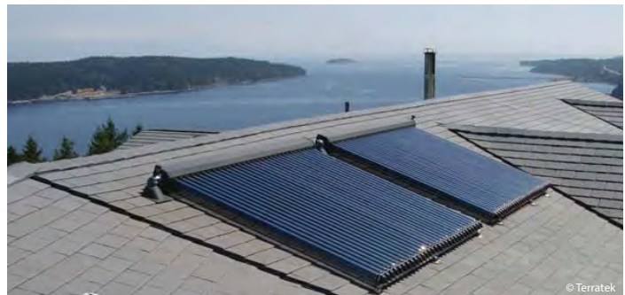
Two evacuated tube collectors.
