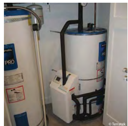
Solar hot water tank (r) with a pump station and external heat exchanger attached.
