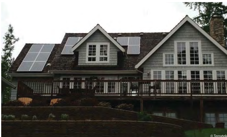
Three kilowatt solar photovoltaic system, with battery back-up, installed in Fanny Bay, BC.
