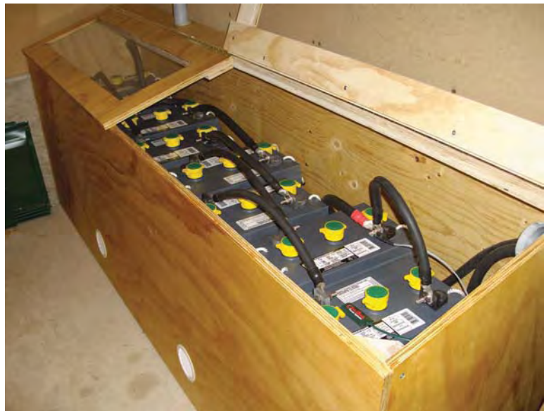
10 kWh battery bank for residential solar grid-tie with battery back-up.
