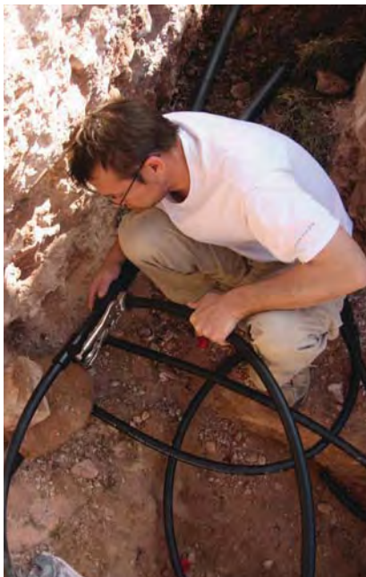
Horizontal trench manifold.
