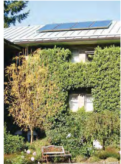
Four collector residential solar hot water system.
