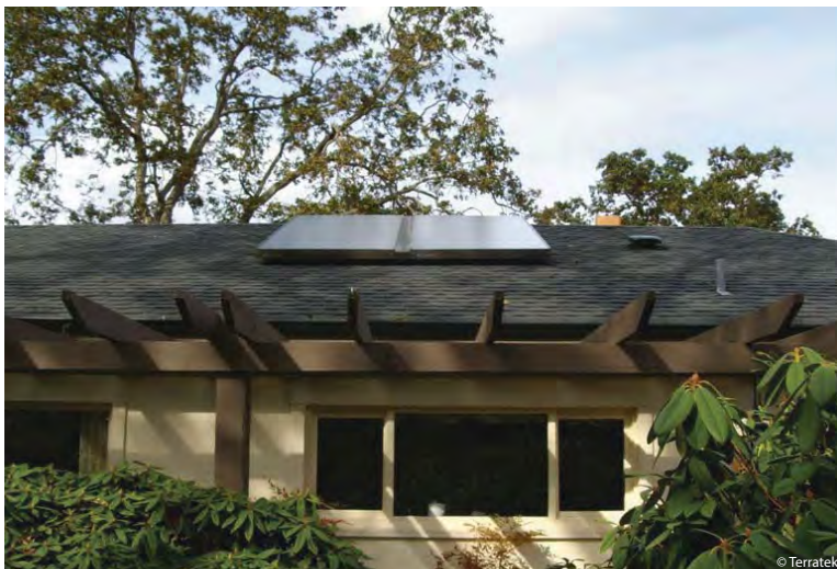
Two flat plate solar hot water collectors on a residential home in Comox Valley.
