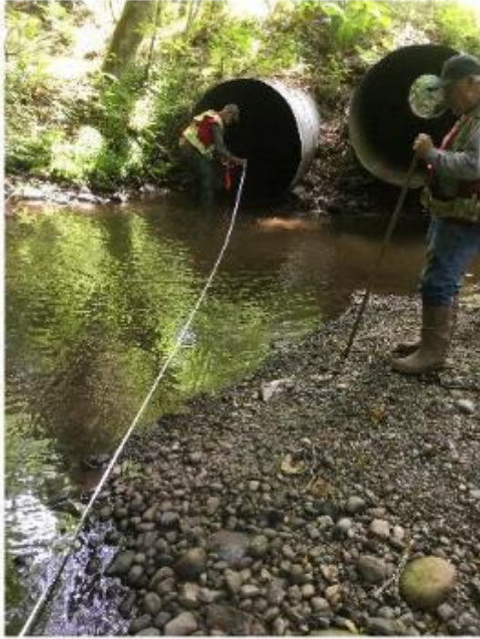
Photo 1) Reach 2, Bradshaw Road culverts hung and rotten
