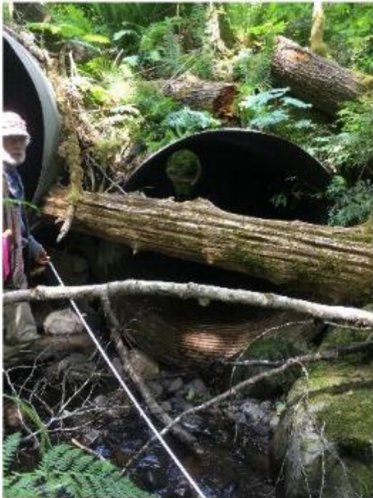
Photo 3) Bradshaw culvert impairing fish passage and hydrology
