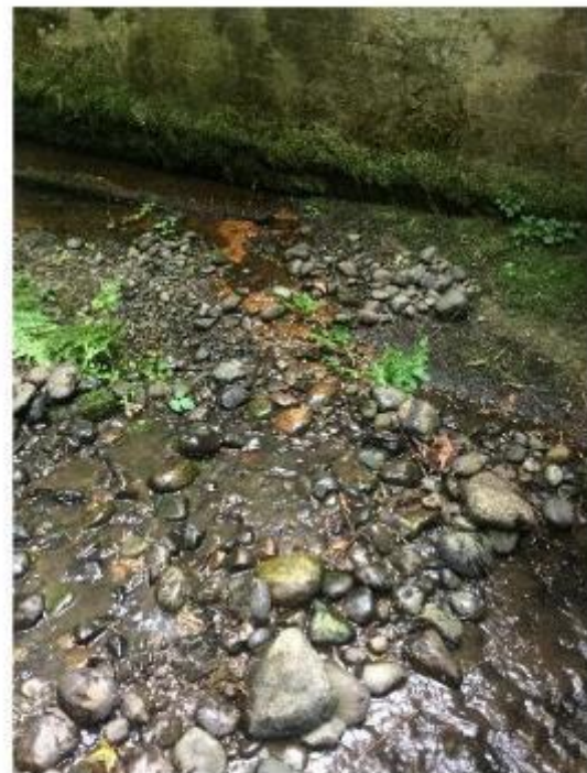
Photo 4) Railway culvert leaching iron residue into creek
