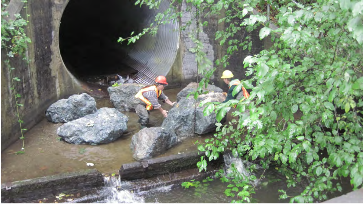
Photo 16. Installation of over-sized boulders using 30 ton boom truck at Highway 19A culvert in Thames Creek.
