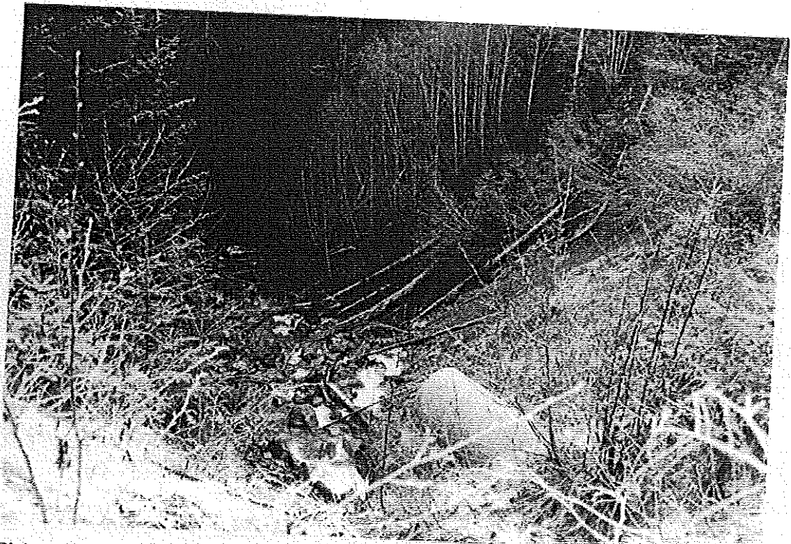
Plate 17. Stop #8. Looking downstream at Yellow Creek from Cameron Main. Two culvert pipes visible.
