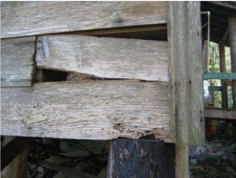
Severe structural deterioration shown in Craft Hut Building
