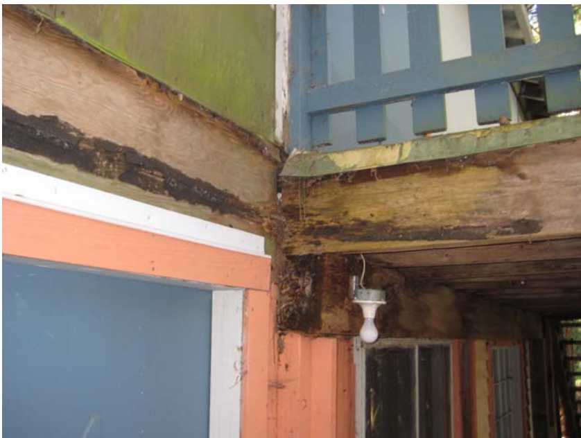
Structural deterioration of balcony and siding at Stringer Hall
