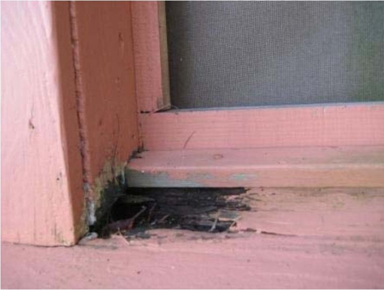
Rot and decay are evident in many parts of the older cabins. Shown in windowsill here.
