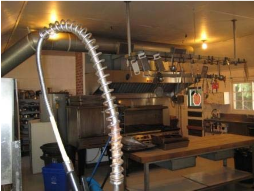
Commercial kitchen in Stringer Hall
