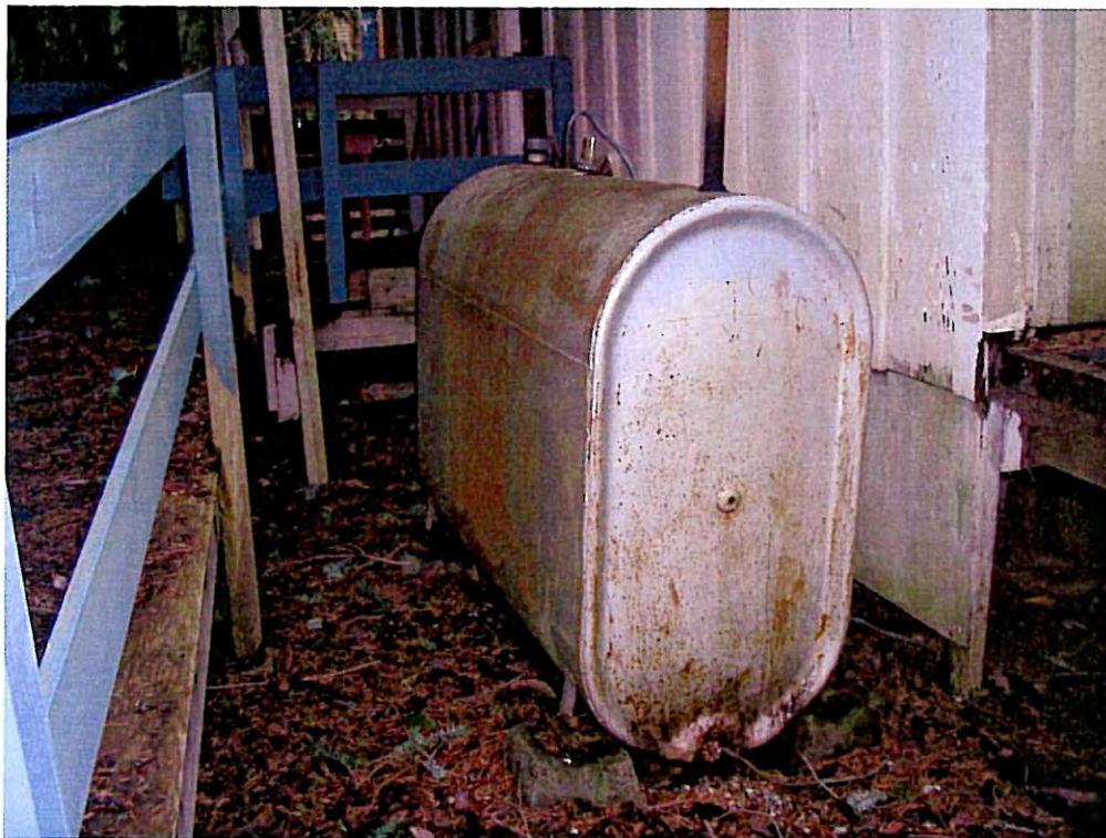
4. Heating oil tank on east side of Splash 1 building.
