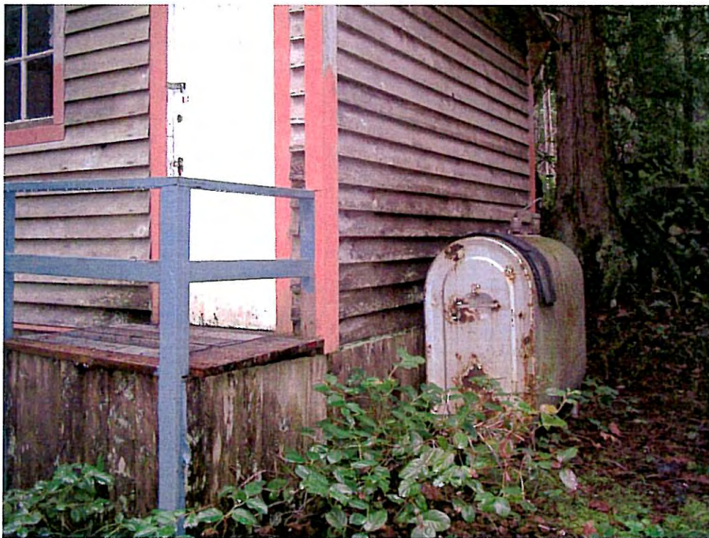
2. Fern Cottage with typical older 275 gallon furnace oil tank.
