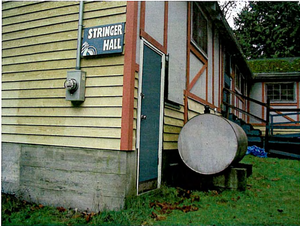
1. Despite its age, the furnace oil tank by Stringer Hall is in good condition.
