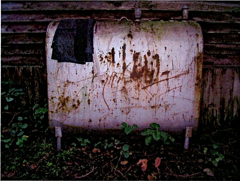
Figure 5. Flaking paint was noted on the furnace oil tank for Fern Cottage.
