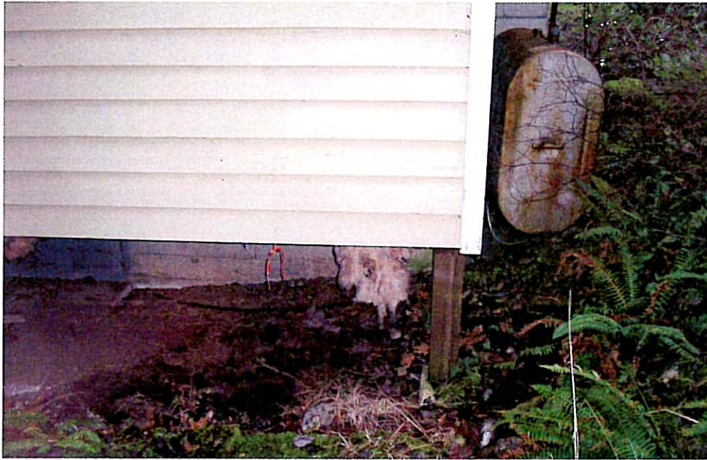
3. Heating oil tank located behind Caretaker's Residence.
