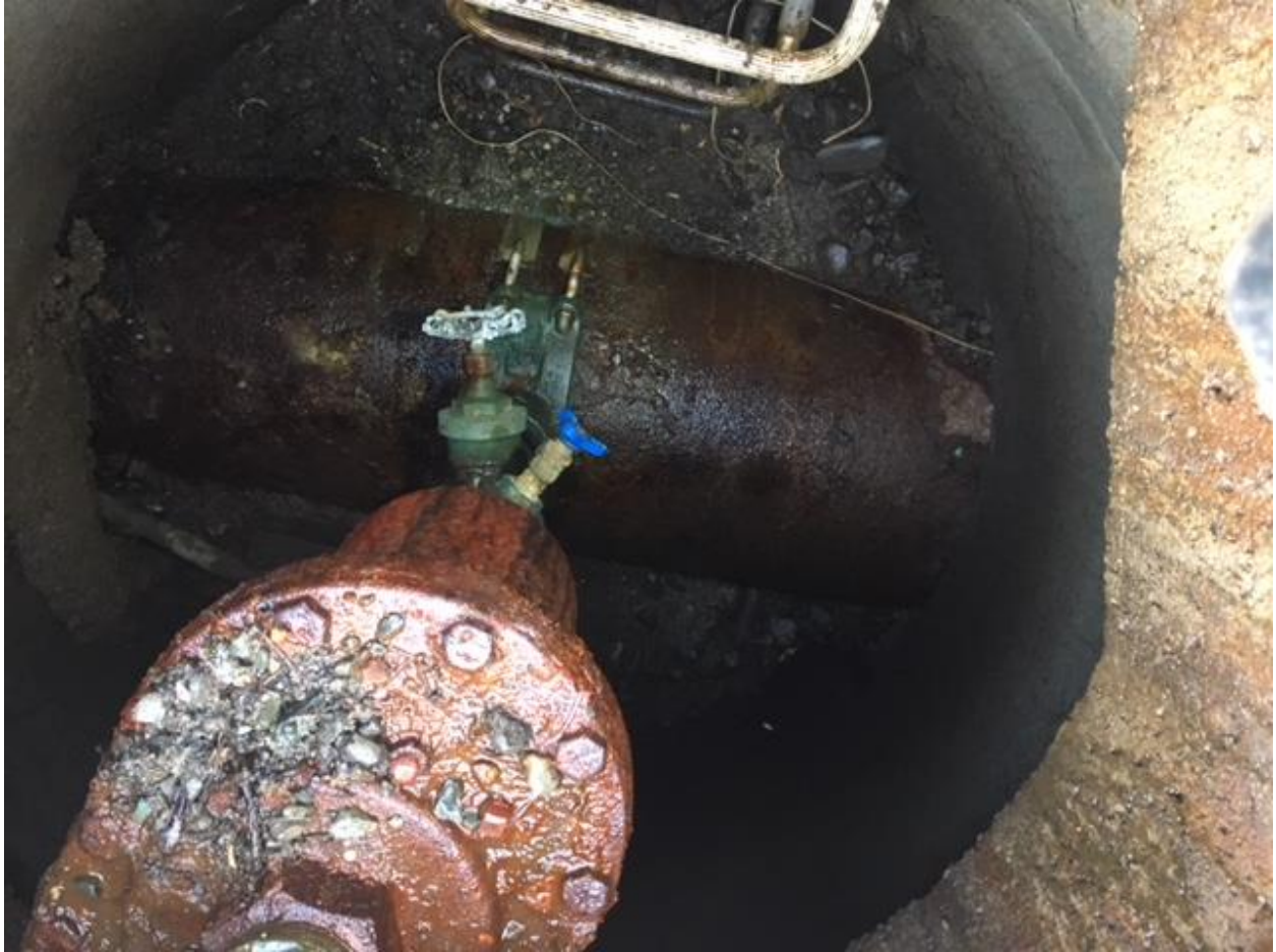
Air valve on ductile iron transmission main at the corner of Northwest Bay Road and Claudet Road
