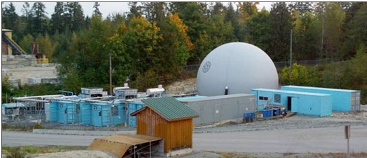
Figure 16-2 Cedar Road Bioenergy Landfill Gas Utilization Plant at the Regional Landfill
