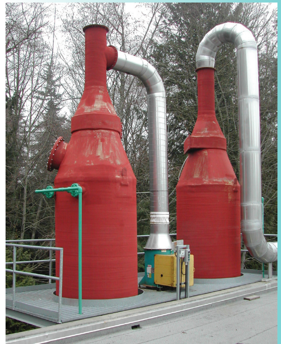
FOUL AIR SCRUBBERS AT FRENCH CREEK POLLUTION CONTROL CENTRE
