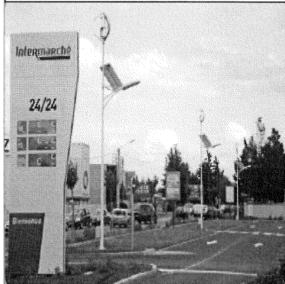
Illustration 2: Maglev Vertical Axis 600W 24V Wind Generator installed in commercial setting
