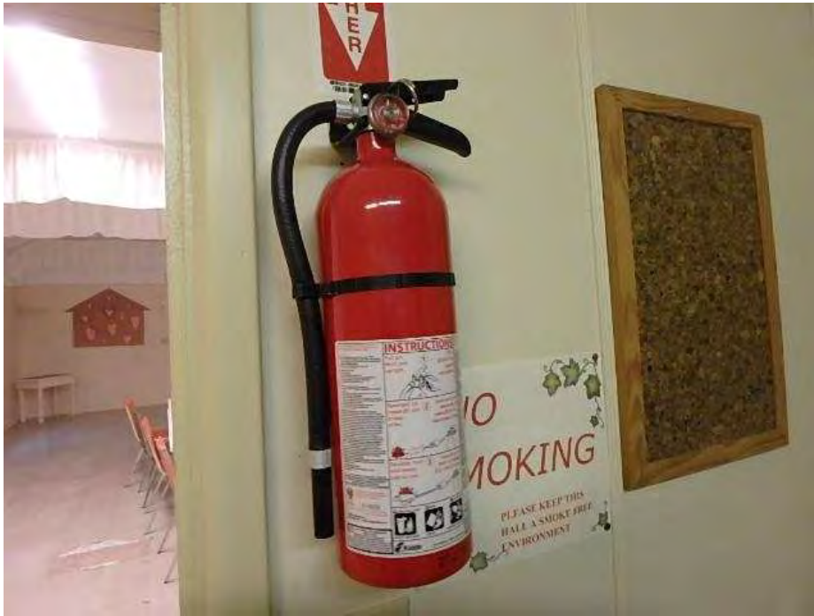
Extinguisher due for service
